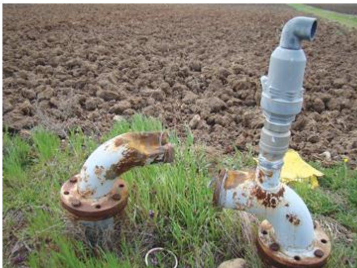
Image 6 Broken valve from a pumping station
