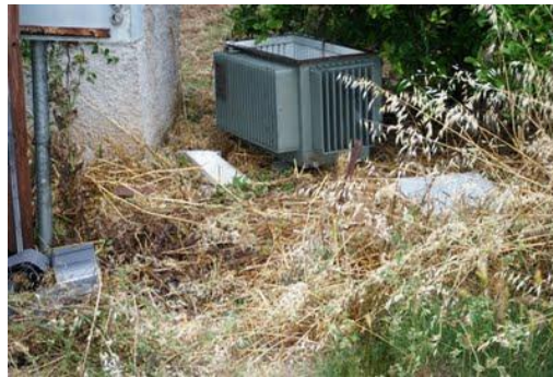
Image 5 Shell of broken transformer
