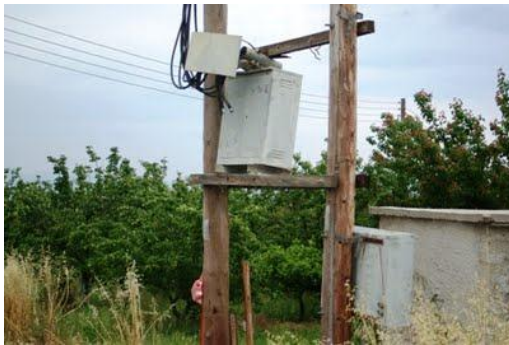
Image 4 Shell of broken transformer
